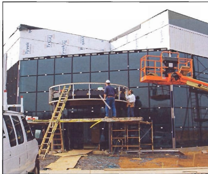
Photo by Jim Marsh Work progresses on the Metro School of Cosmetology under construction in Wescosville.
